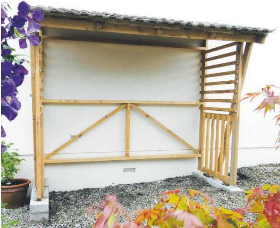
The diagonals on the back are pieces of roofing baton tightly cut into the frame. They triangulate the back, providing a sudden and startling rigidity to the whole structure
